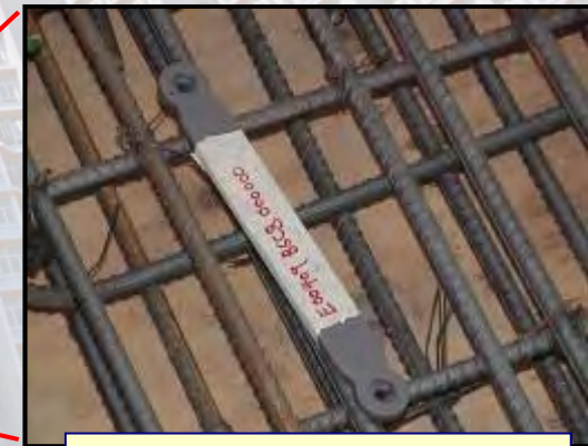
RFID Tag installed inside the facade
