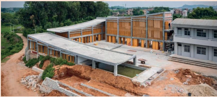
The construction work was at the final stage, and will be completed by October.
