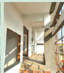
The wooden façade will be installed and the internal renovation works will commence afterwards.
