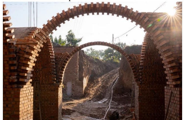
Brick panels were placed at the sides of the arches, and curved steel bars were added to provide structural integrity.
