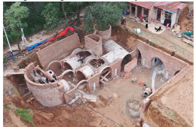
The construction works to revitalize the silo-cave were in process on site.
