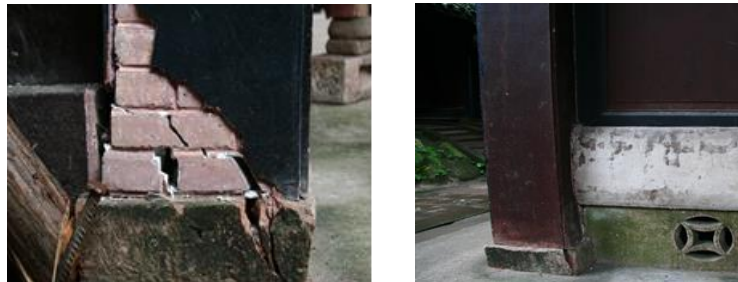
Fig.16 Actual earthquake damages of brick/stone columns
