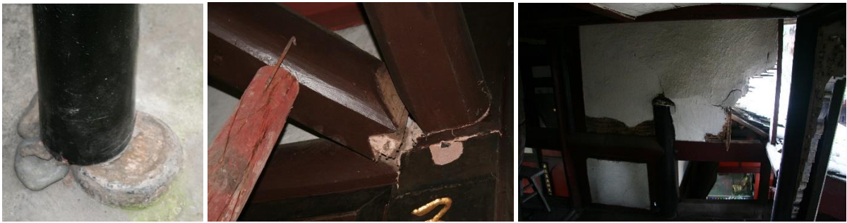
(a) column foot movement (b) tenon pull-out (c) maintenance walls damage
