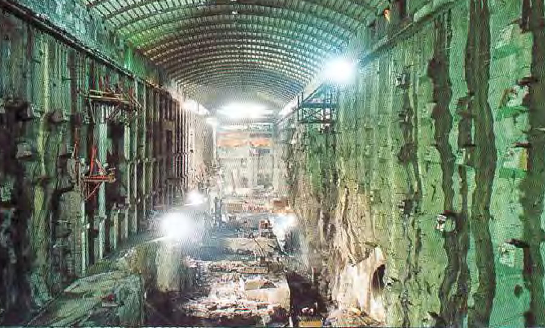
Er Tan Underground Power House
