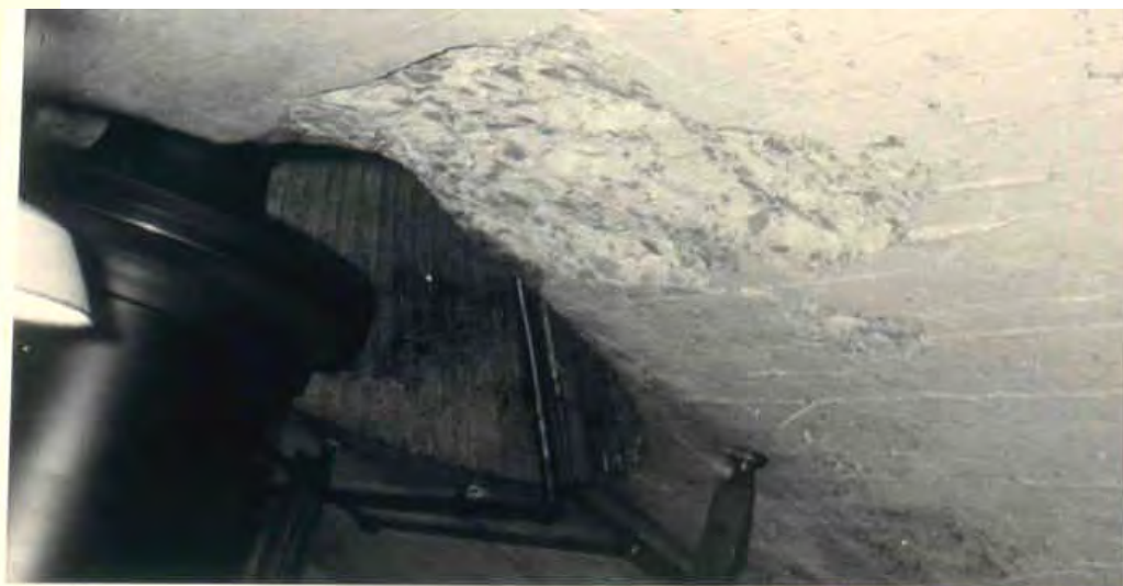
FIG. 4-1 Wheel Pit, Lower Arch No. 11 Spalling, underside, south half
