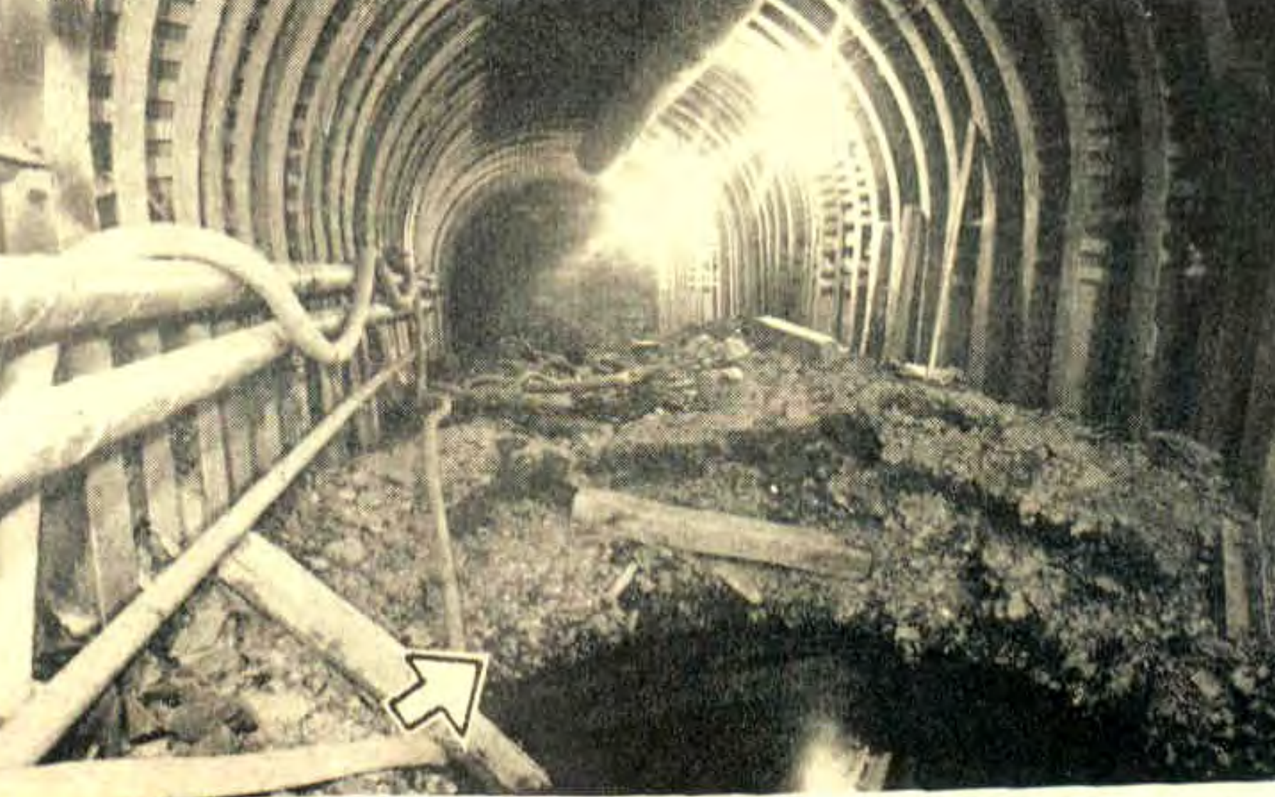
LEAVED —Shale moved up into cross-section requiring invert re-excavation
